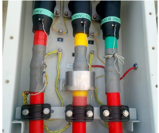
Existing supplied electrical equipment photograph.
